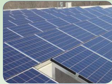
Provision for future solar panels to target reduced energy costs & reduced reliance on fossil fuels.
